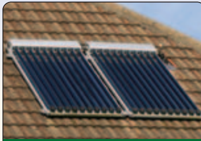
Apricus solar collectors convert energy from the sun into usable heat.
